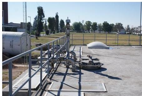
Output of biogás from UASB anaerobic reactors
