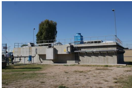
UASB anaerobic reactors
